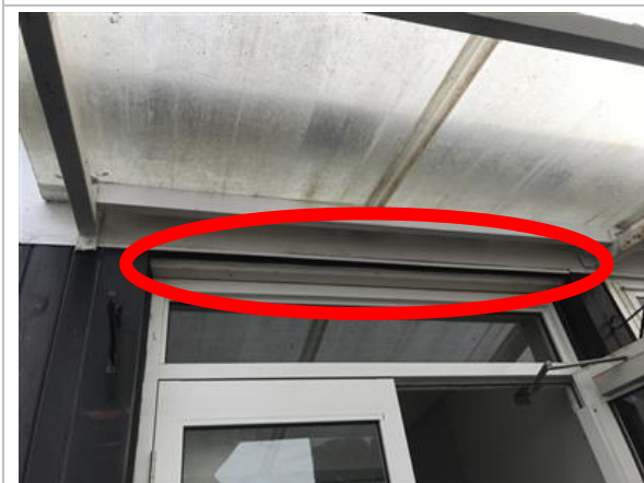
Photograph 39: A gap between the top of the wooden door frame and the wooden fascia chip board on is on the west face of Building 5 with Low suitability to support roosting bats (Figure 1: F5a).
