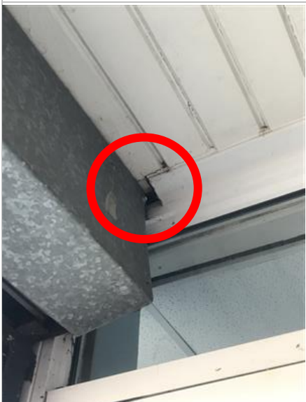
Photograph 43: A hole in the corner of the roof near metal shutters on northern face of Building 11 with Low suitability to support roosting bats (Figure 1: F11a).
