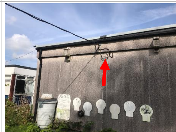
Photograph 40: Location of a gap behind the fascia/vent on the west face of Building 8 approximately 2.5 m above the ground with Low suitability to support roosting bats (Figure 1: F8a).
