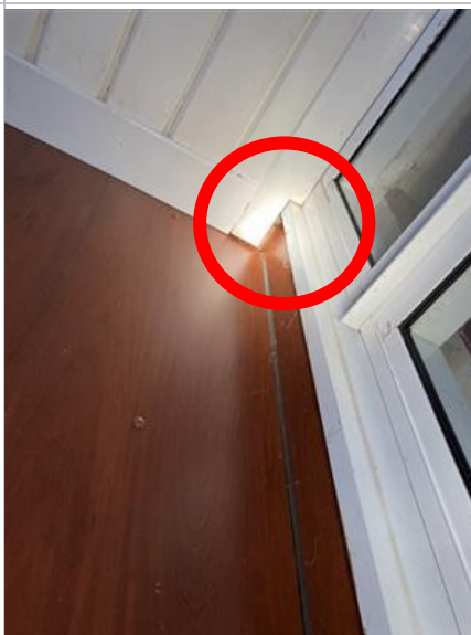
Photograph 44: A gap in the corner between the northern face of Building 11 and the eastern face of Building 10, approximately 2.5 m above the ground and between the wooden wall and window adjacent to end of a soffit board (Figure 1: F11b).
