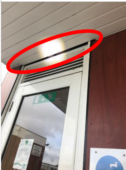
Photograph 34: A gap with Moderate suitability to support roosting bats on the north face of Building 2 above a doorway (Figure 1: F2a).
