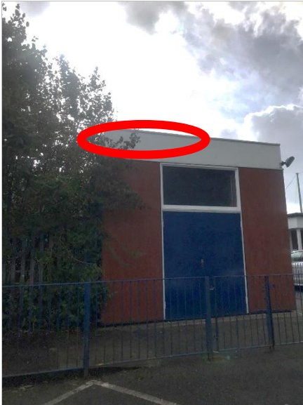
Photograph 35: Location of a gap under the metal roof in the northeast corner of Building 3 with Low suitability to support roosting bats (Figure 1: F3a).
