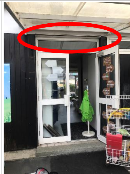
Photograph 38: Location of a gap between door frame and fascia chip board on west face of Building 5 with Low suitability to support roosting bats (Figure 1: F5a).
