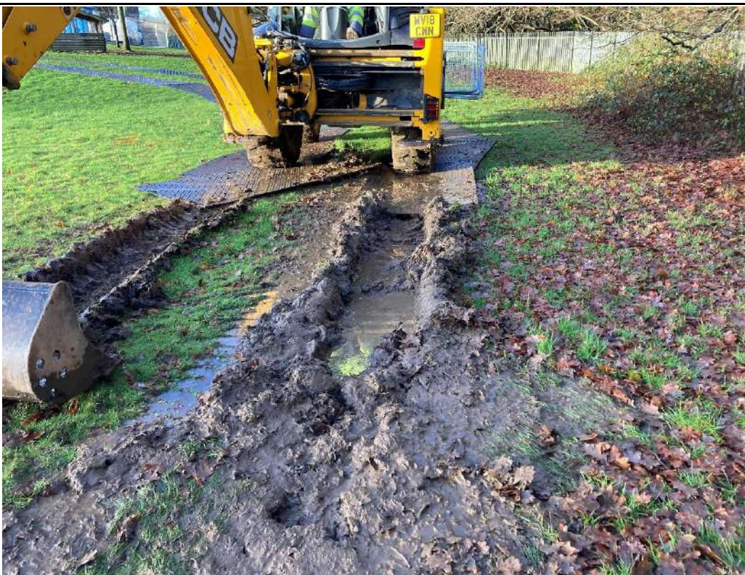
Plate 68 Image of ground disturbance as a result of wet ground during site works
