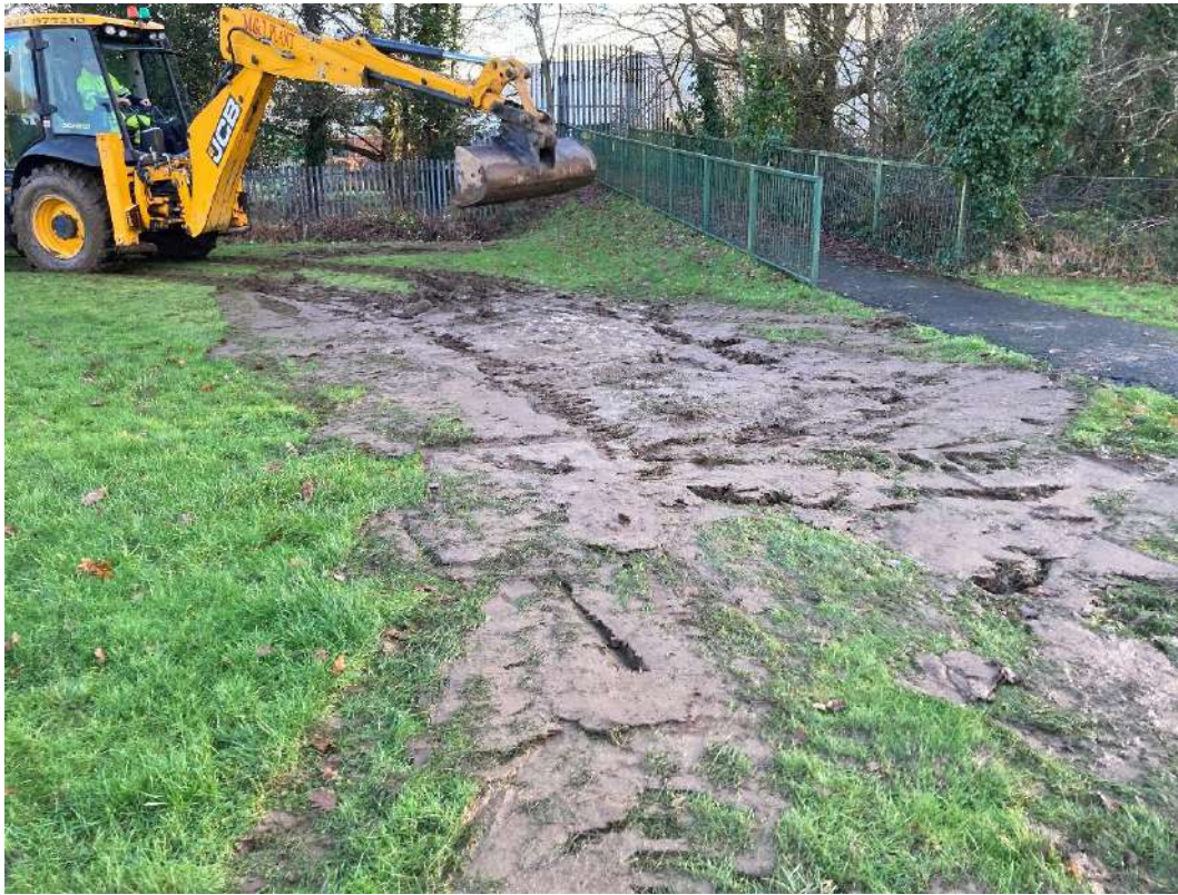
Plate 75 Image of ground disturbance as a result of wet ground during site works, smoothed
