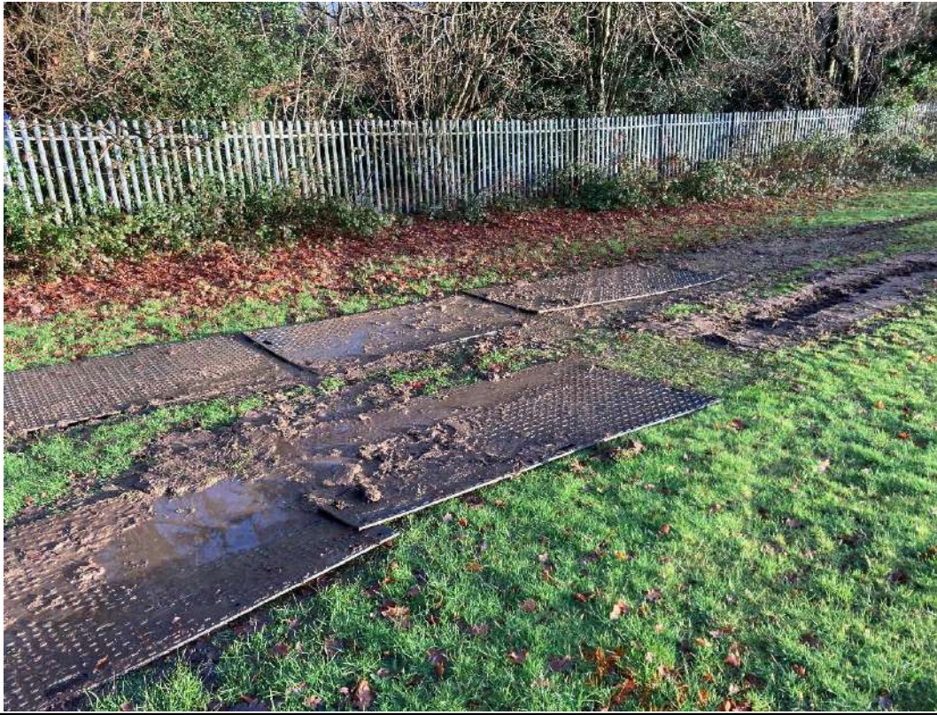
Plate 77 Image of bog mats laid over wettest areas during site works to prevent damage
