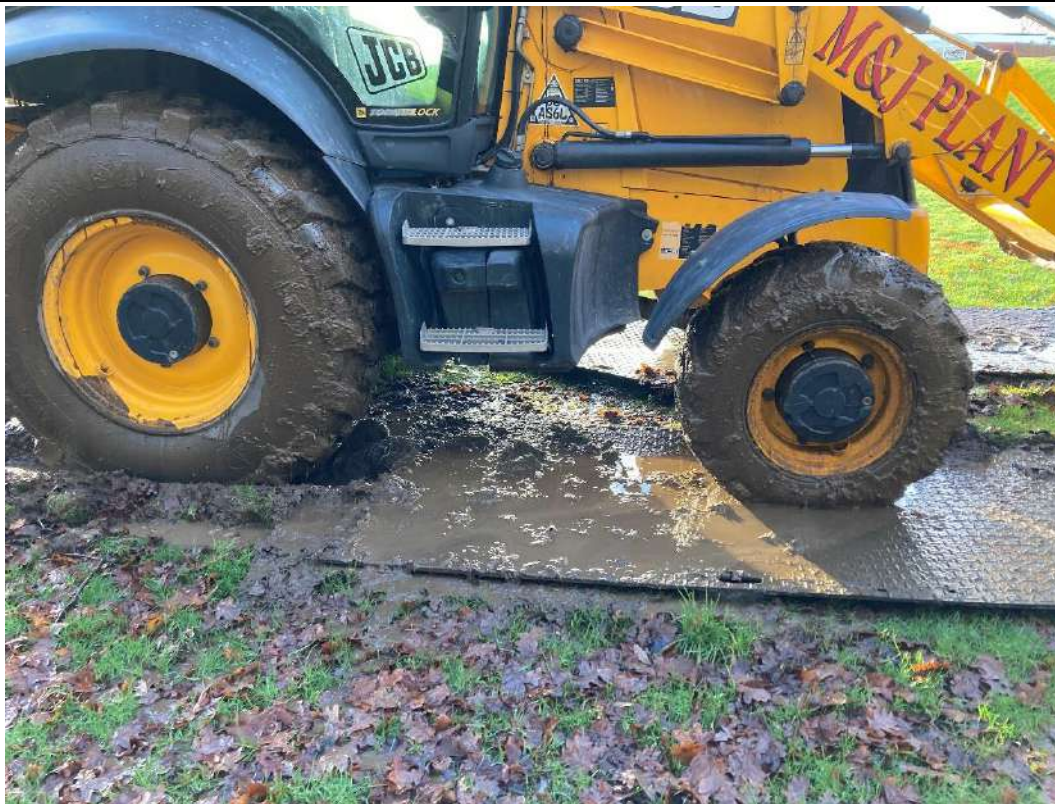
Plate 72 Image of ground disturbance as a result of wet ground during site works and bog mats
