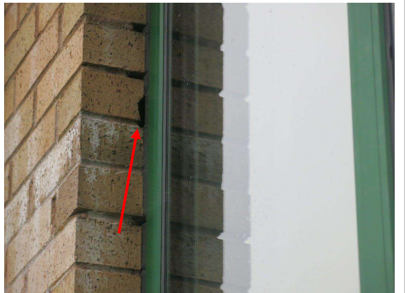
Figure 8.3: Pavilion E – gap between brickwork and window frame
