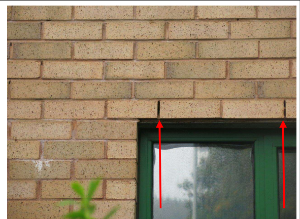
Figure 7.3 Pavilion B – weep holes above window.
