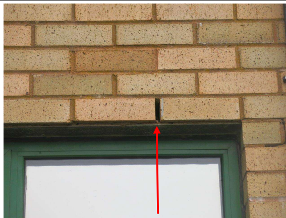
Figure 7.2 Pavilion B – weep hole PRF above window.
