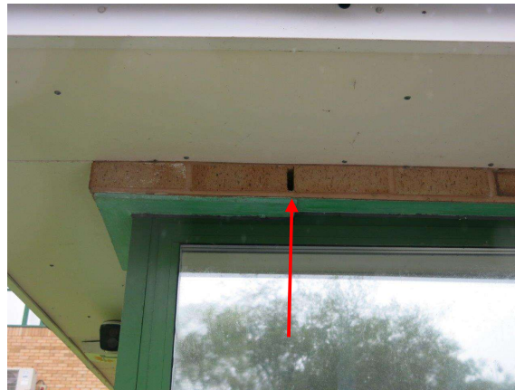
Figure 11.2: Security lodge (north elevation) - weep hole PRF
