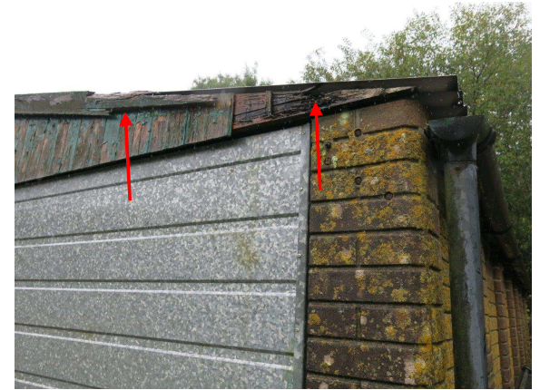
Figure 12.3 Eastern Garage (north elevation) gap behind bargeboard PRF and rotten wood PRF.
