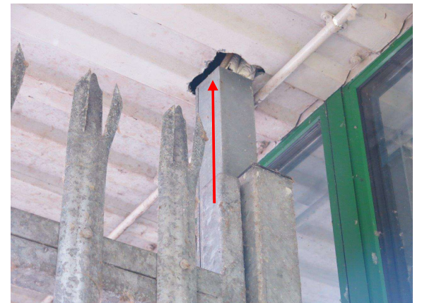
Figure 6.6: Gap in soffit board above metal post in Pavilion C. Not considered suitable for bats a smooth survey would make it difficult for crawling bats to gain purchase.
