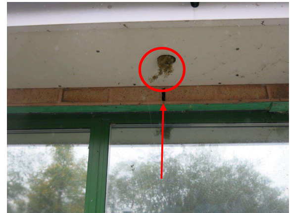
Figure 11.3: Security lodge (west elevation) - weep hole PRF and old bird's nest in soffit vent
