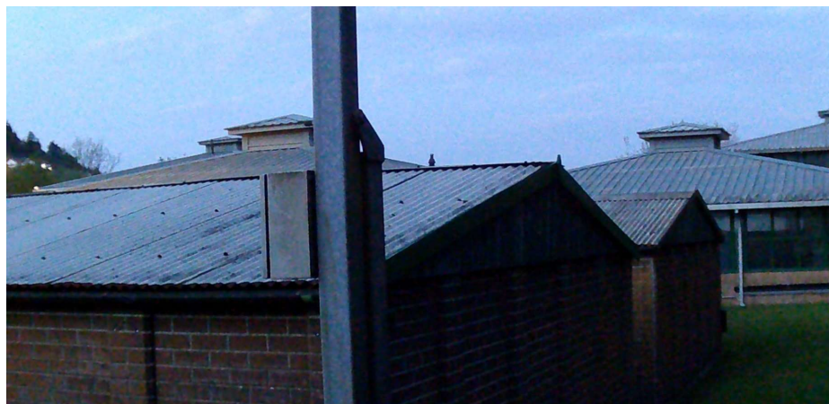
Garages – south and west (part) elevations. IR illumination failed on this camera.
