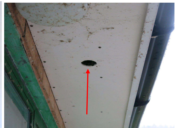
Figure 11.6: Security lodge (south elevation) - soffit vent gap - unused by birds at time of survey.
