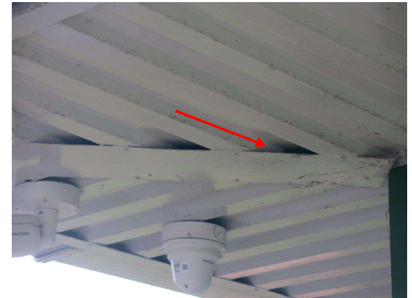
Figure 6.3: Soffit metalwork. Gaps present but not considered suitable for bats due to poor thermal condition and smooth surface making it difficult for crawling bats to gain purchase.
