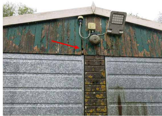
Figure 12.2 Western Garage (north elevation) gap in gable end wooden paneling PRF/access point.
