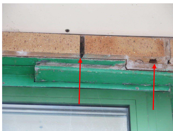
Figure 9.7: Pavilion F (east elevation) weep hole PRF above window – also showing mortar gap PRF.
