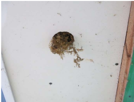
Figure 11.4: Security lodge (west elevation) close-up of bird's nest in soffit vent gap.
