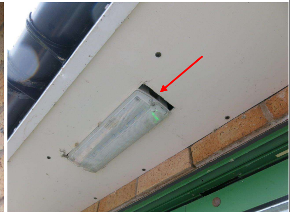
Figure 9.9: Pavilion F (east elevation) gap by light - potentially used by birds as nest site although artificial light may deter birds (and bats) from using.
