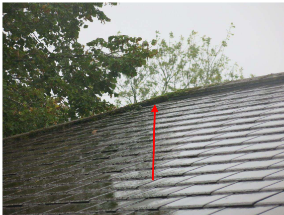
Figure 9.4: Pavilion F (west elevation) PRF where mortar has come away from beneath ridge tile.
