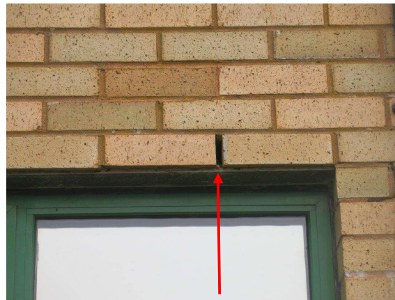
Figure 6.2 Pavilion B – weep hole PRF above window.
