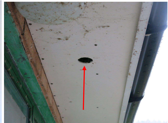
Figure 10.6: Security lodge (south elevation) - soffit vent gap - unused by birds at time of survey.
