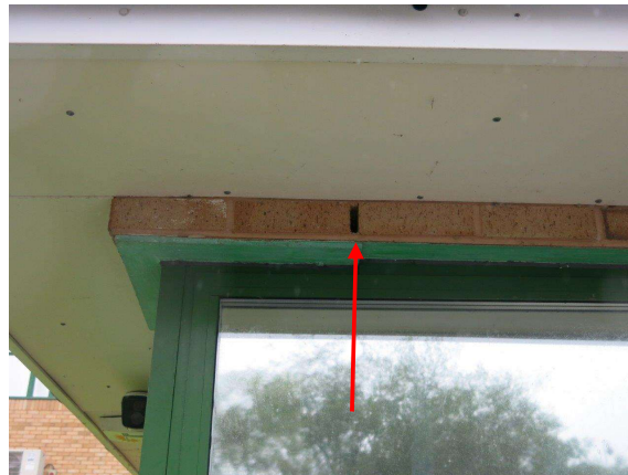
Figure 10.2: Security lodge (north elevation) - weep hole PRF
