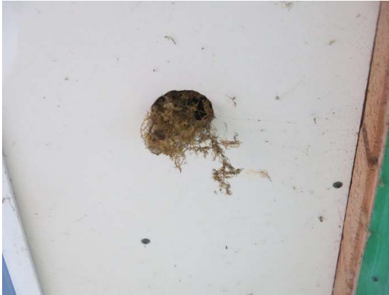
Figure 10.4: Security lodge (west elevation) close-up of bird's nest in soffit vent gap.
