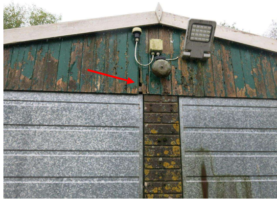
Figure 11.2 Western Garage (north elevation) gap in gable end wooden paneling PRF/access point.
