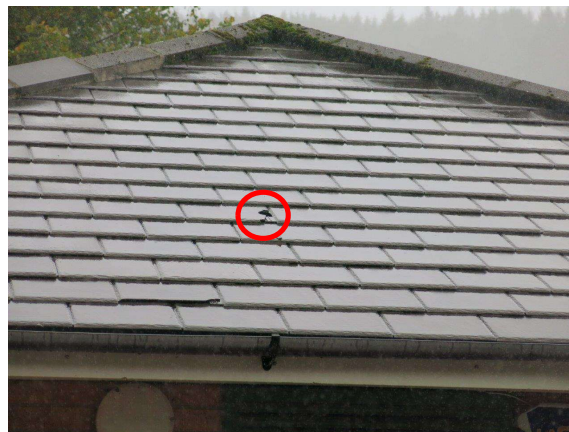
Figure 8.2: Pavilion F (south elevation) broken roof tile PRF
