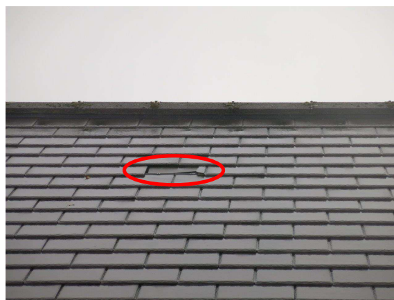
Figure 8.5: Pavilion F (west elevation) damaged roof tile PRF.
