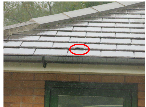
Figure 8.3: Pavilion F (south elevation) gap under roof tile PRF.
