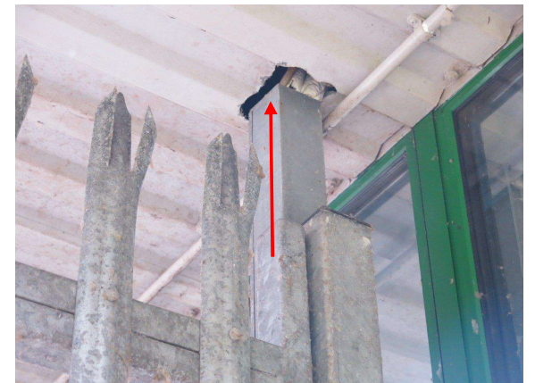
Figure 5.6: Gap in soffit board above metal post in Pavilion C. Not considered suitable for bats a smooth survey would make it difficult for crawling bats to gain purchase.
