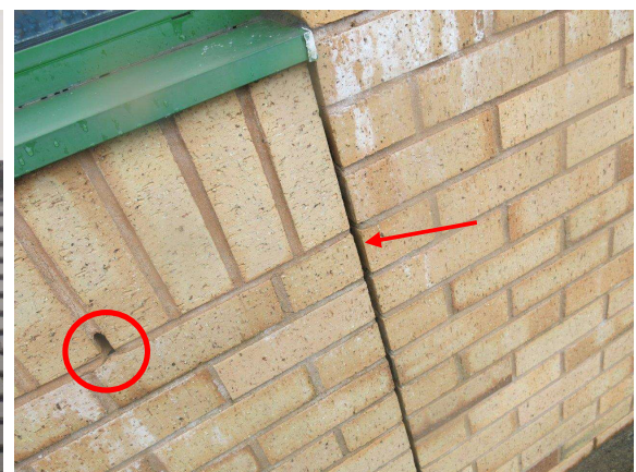
Figure 8.6: Pavilion F (east elevation) weep hole PRF below window and brickwork gap PRF.
