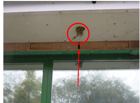
Figure 10.3: Security lodge (west elevation) - weep hole PRF and old bird's nest in soffit vent
