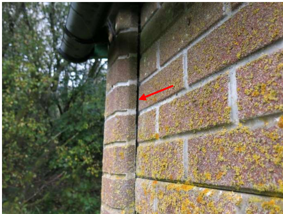
Figure 11.4: Eastern Garage (east elevation) brickwork gap PRF.
