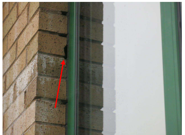
Figure 7.3: Pavilion E – gap between brickwork and window frame
