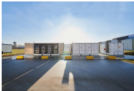
Figure 4 An example battery storage facility.
