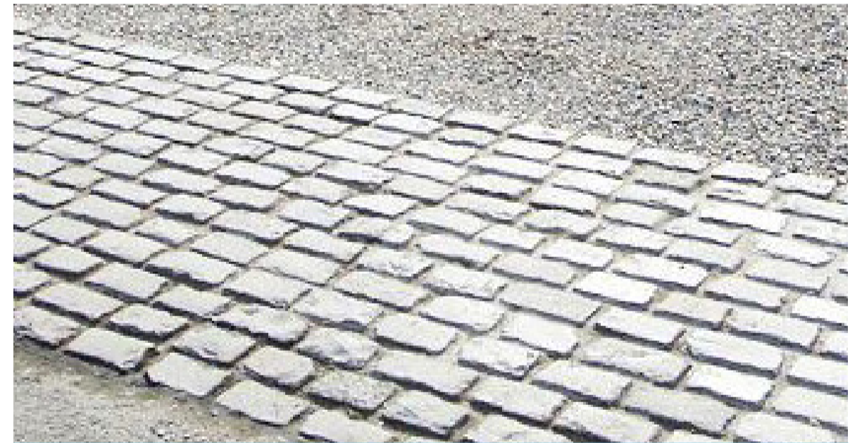
Public Realm 3C - Cobbled Crossing: Traditional-style cobbled stone has been used within the village as a surface treatment. The cobbles can be used as part of the pedestrian crossing design as a tactile material which would define the extent of the crossing area.
