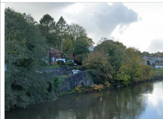
Photograph 9: Southeast bank in upstream section of the Survey Area. Bank is made of concrete and boulders (Figure 1 and Appendix A: TN 5).
