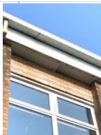
Photograph 6: Building elevation: B2c, PRF: B2c_Ref_01. South elevation of building. loose soffit panel with gap underneath. Emergence of two common pipistrelle confirmed from this feature on 08.09.2022.
