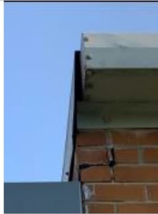
Photograph 8: Building elevation: B2d, PRF: B2d_Ref_01. On west elevation of building. Gap at corner of soffit/ flashing/roof capping.
