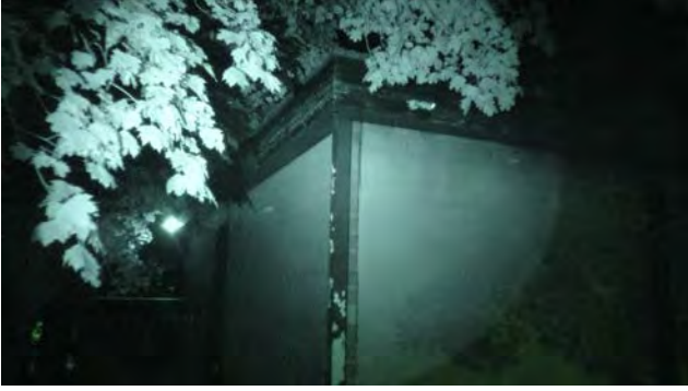
Photo 7. The eastern and southern elevations of the workshop at the darkest point of the survey on the 20 th September 2022.
