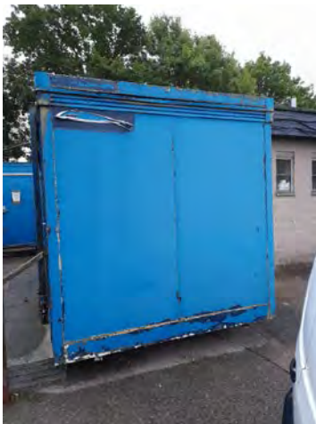
Photo 34. The western elevation of one of the temporary buildings located in the eastern section of the site.
