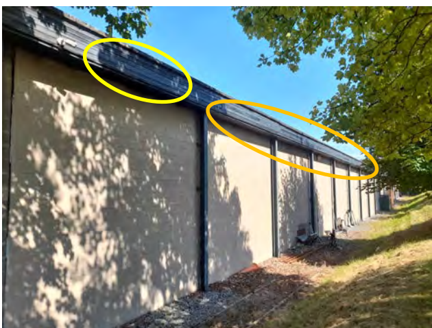
Photo 36. The eastern elevation of the workshop with the common pipistrelle (orange) and soprano pipistrelle (yellow) access features highlighted.
