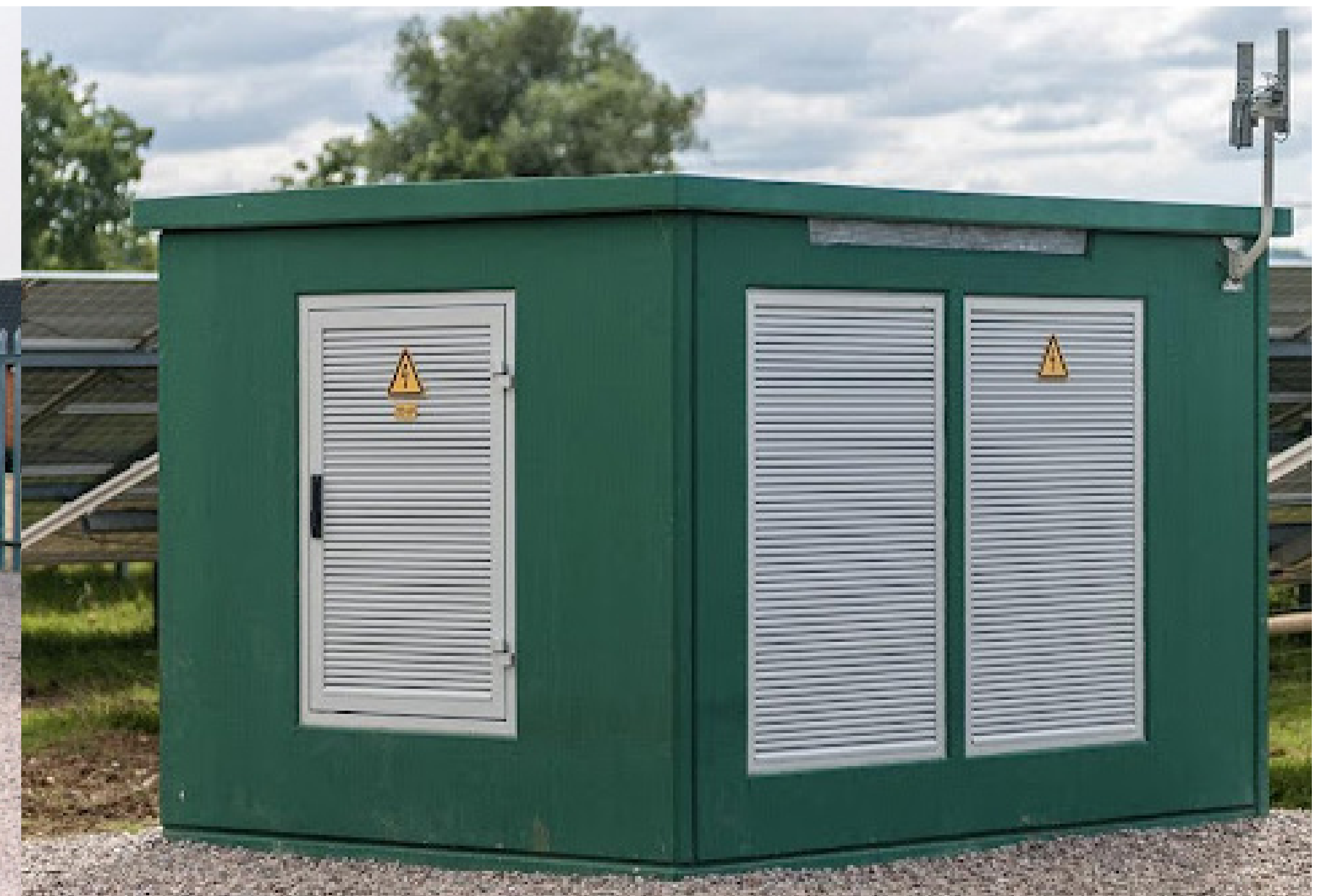
Is-orsafoedd Cwsmeiriad ac Ysbyty/ Customer and Hospital Substations
