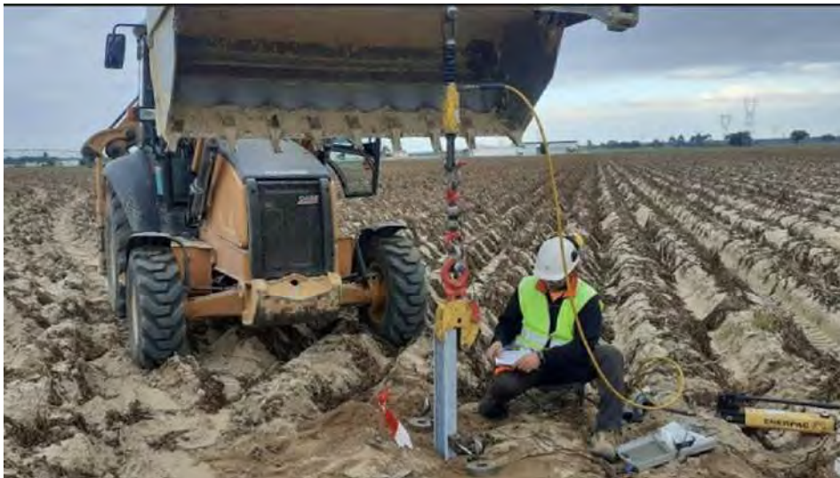
Figure 2.2: Axial load testing for solar PV array using a driven steel section pile. Ref: elaborex@elaborex.es
