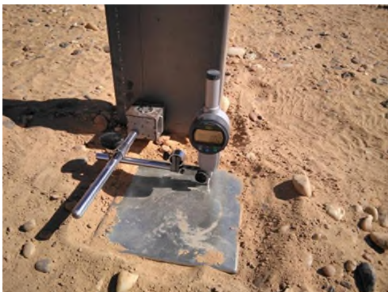
Figure 2.3: Micrometer installed for measuring the displacement of the section during lateral load test. Ref: Camara J, Marin F. Technical Specifications for the Realisation of Static Load Tests for the Foundation of Photovoltaic Plants (Undated Online Paper).
