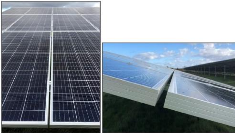
Figure 8. Photovoltaic Panel Gaps
